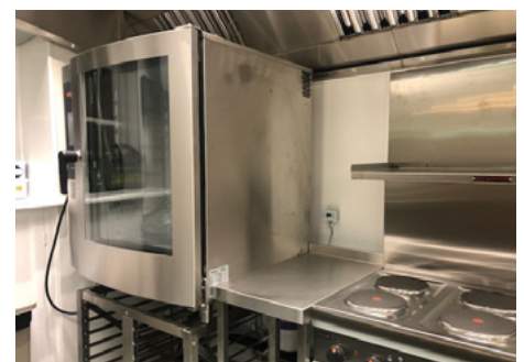
Some of the serious catering equipment.
